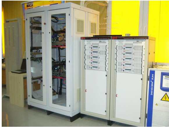
Figure 2. 25kW (2×12.5KW) grid connected PEM fuel cell in Taleghan
